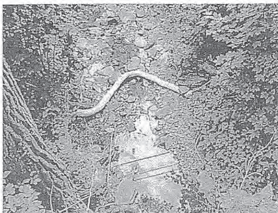
Above: A baffle installed in a tributary of the Esopus Creek near the chemical spill at William Hrazanek's Wittenberg Road property in Mount Tremper. Photo taken on July 11 by Julia Reischel.
